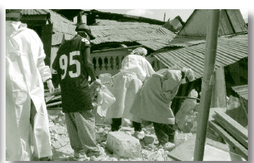
Hospital workers dig through rubble at the St. Francois de Sales hospital in Port-au-Prince, Haiti on Friday, January 15, 2010 in the aftermath of the 7.0 magnitude earthquake that struck earlier that week.
